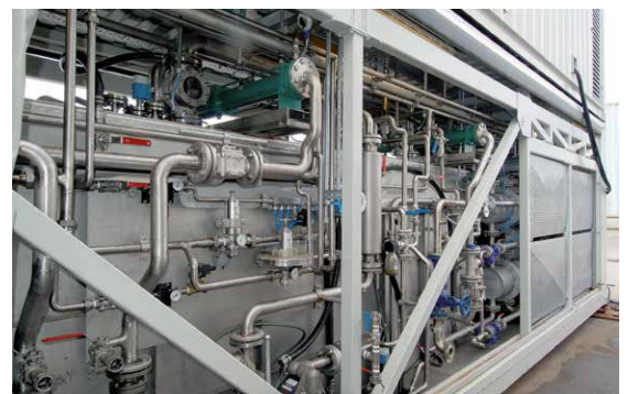
A complex system of pipes with an integrated heat exchanger
